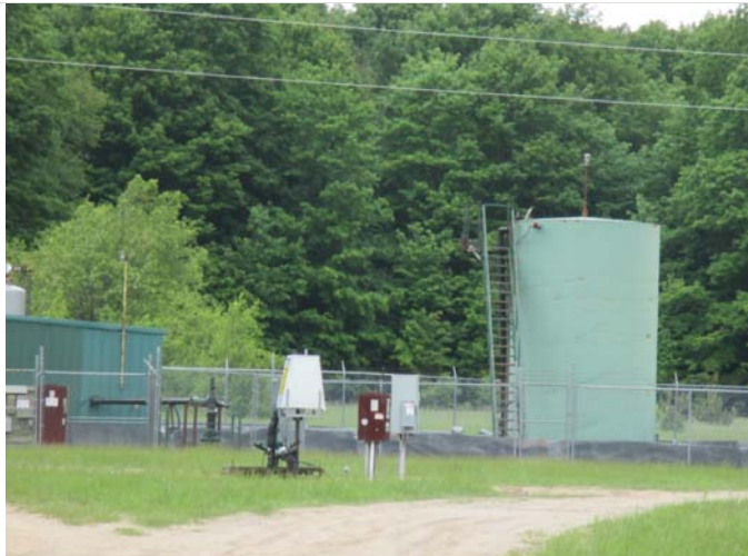
9. A view of brine storage and brine injection well on property south of the site.
