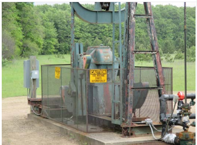
6. A view of natural gas well C1-3 on the northwest portion of the site.
