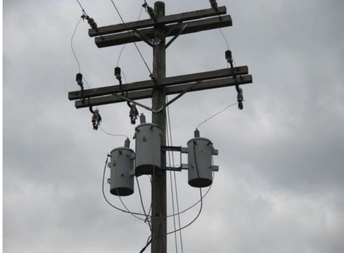
7. A view of transformers near the C1-3 well site.
